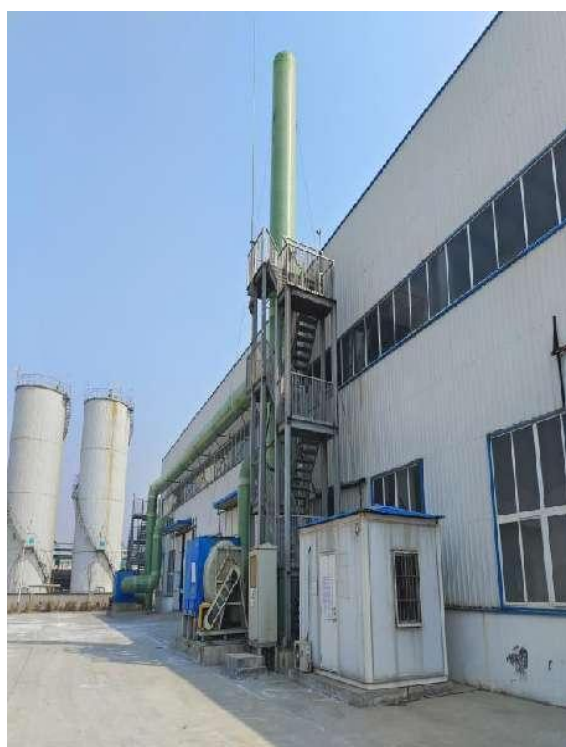
拆包破碎废气 DA008
